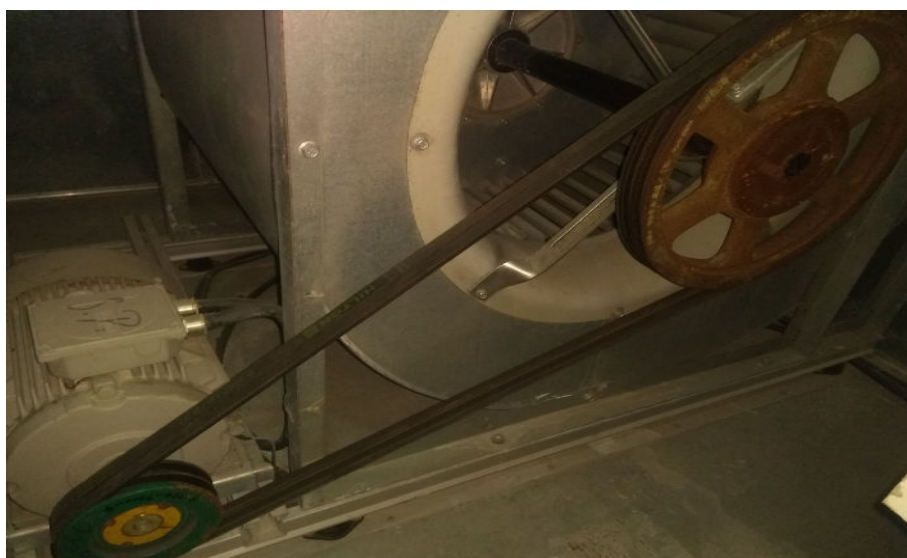
Figure 5:V belt in AHU
