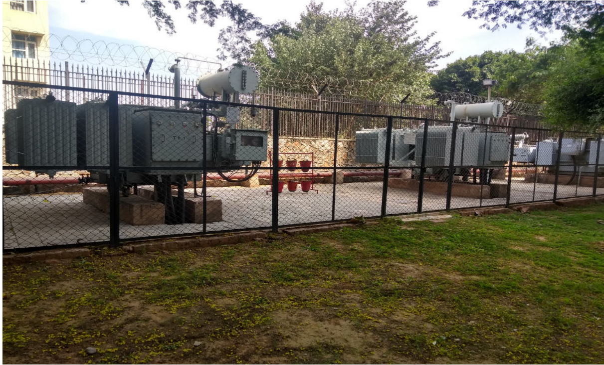
Figure 1:Transformer at Munjal University
