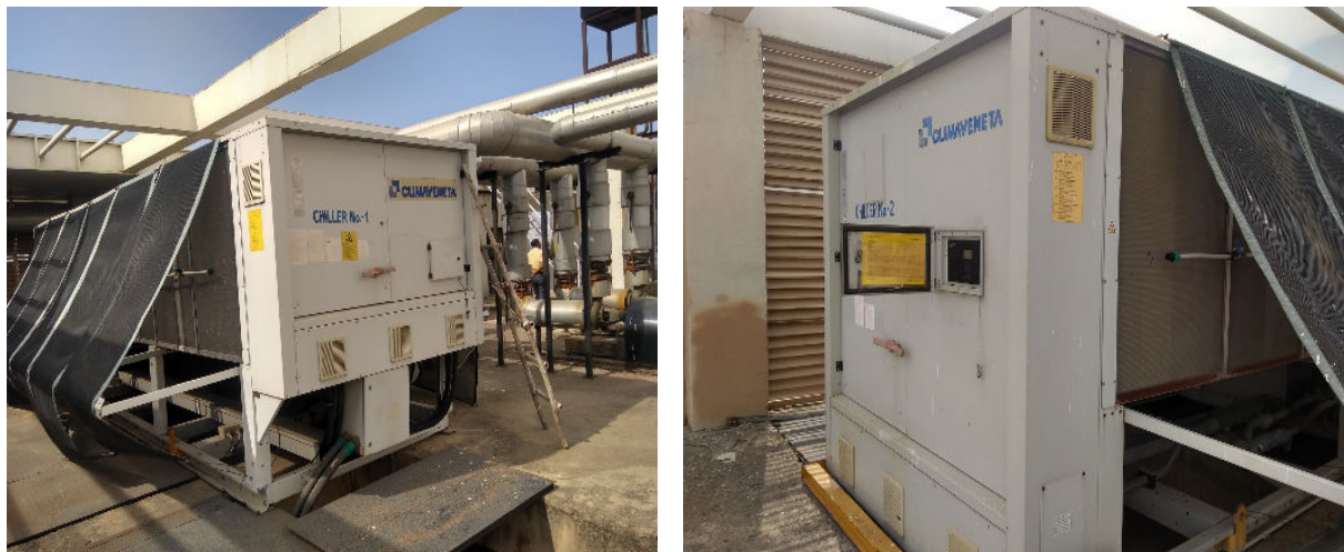
Figure 3: Chillers installed at Elin
