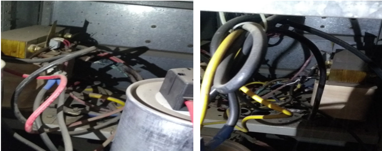
Figure 2:Burnt wires in APFC panel
