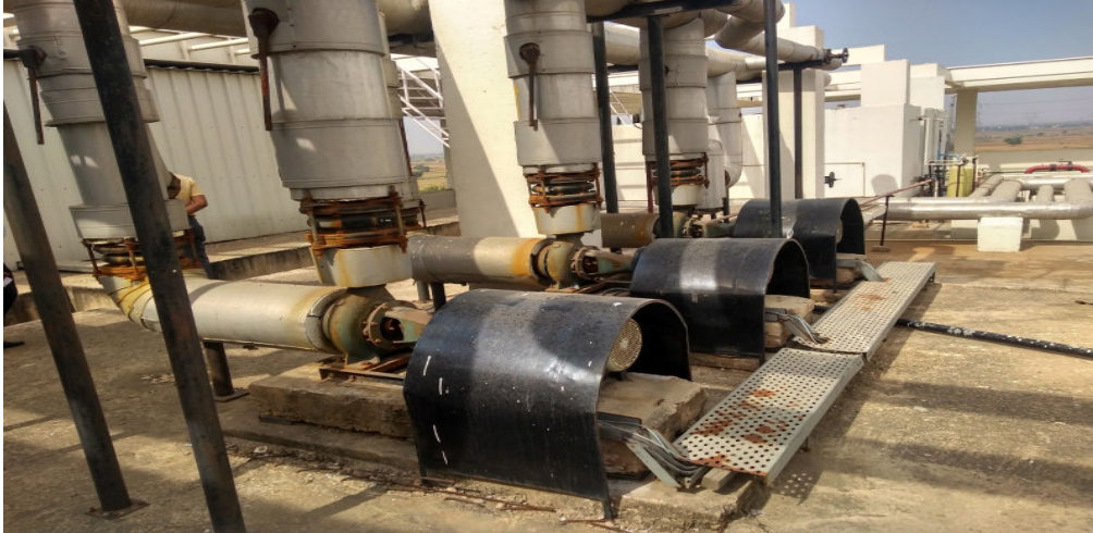
Figure 4:Chilled water pumps
